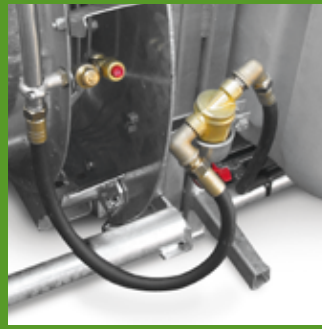
Batch filters before the nozzles
